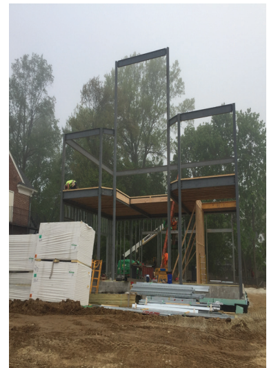
Construction at our new Wayne location is flying along, as you can see the outline of our branded tower.
