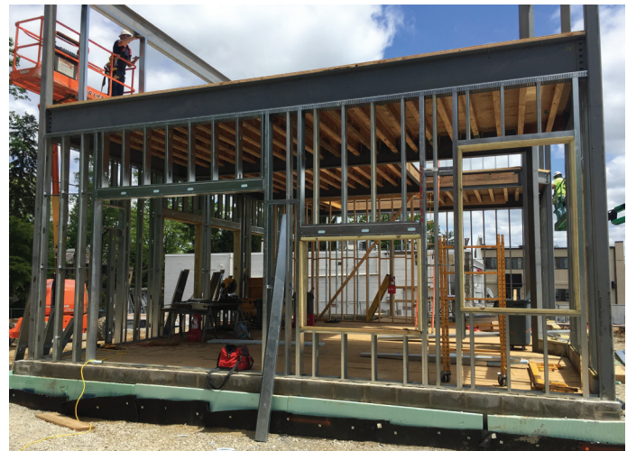
Construction is progressing nicely at our new Wayne location, check out the outside view of our drive-up window!
